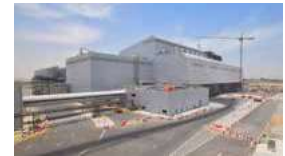
Dubai Waste Management Centre
