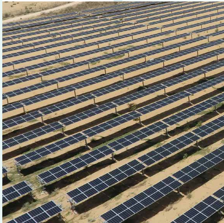
SBSR Solar Project
