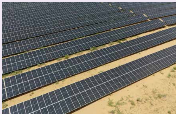
SBSR Solar Project
